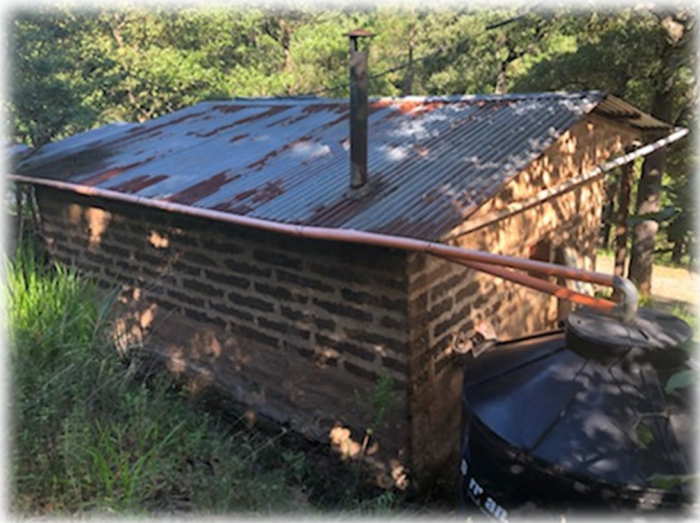
Rooftop rainwater collection system at the Barbara Ford Center
